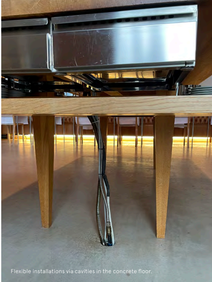
The utilities can be reached by removing a wooden plank along the interior wall of each office.
